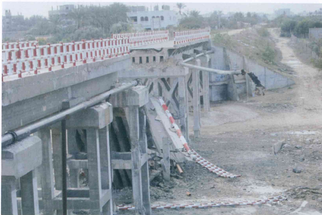
AL Sikka Bridge (After Damaged)
